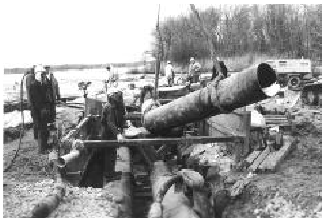
Damaged section of 24 inch pipeline is being removed from a former wooded area on the edge of the impoundment, while workers in background continue to work on extracting oil spilled into the ground and water (2/12/00).
